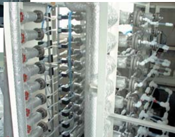
High temperature test line
